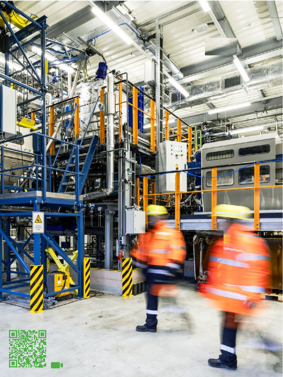
Inside the demonstration plant, engineered in-house, at the Hamburg site.
